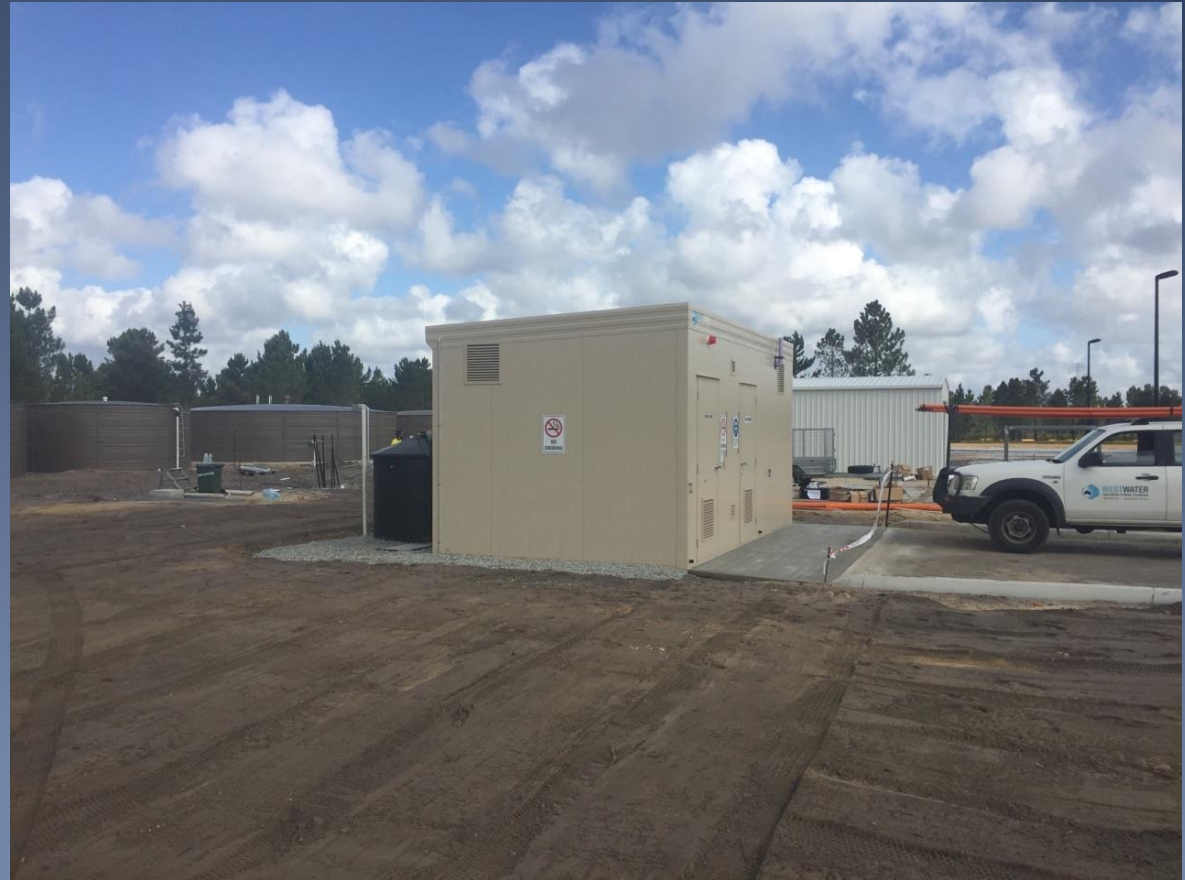
Water treatment module by West Water Pty Ltd
